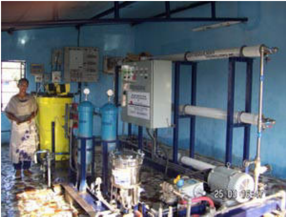
The reverse osmosis plant started operation as soon as it was acquired.
